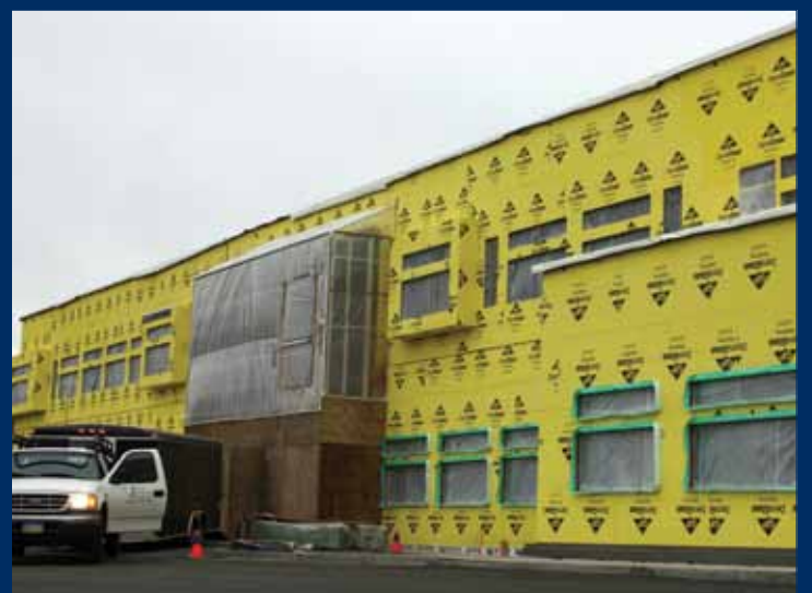
Construction at 11500 C Street progresses on schedule into the winter season. Photo taken on Oct. 25, 2010.
