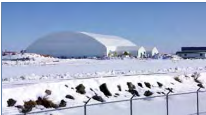
North Wind Services begins construction on a hazardous waste retrieval structure in Idaho.
