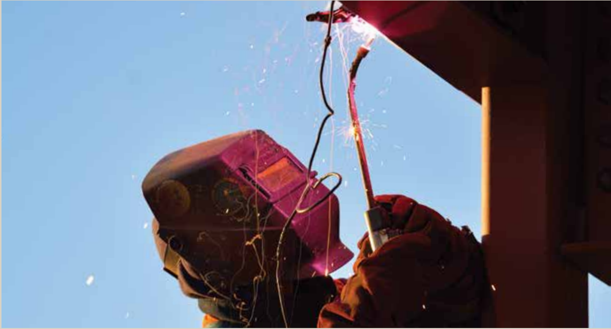
› The SABER contract awarded to Silver Mountain will entail property maintenance, repair and non-complex construction work. Photo by Jason Moore.
