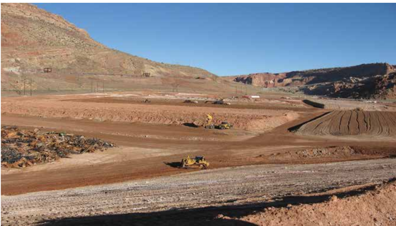
➤ Portage serves as the remedial action contractor for a project in Moab, Utah, which involves moving 16 million tons of uranium tailings to a permanent disposal site 32 miles north. Photo courtesy of North Wind.
