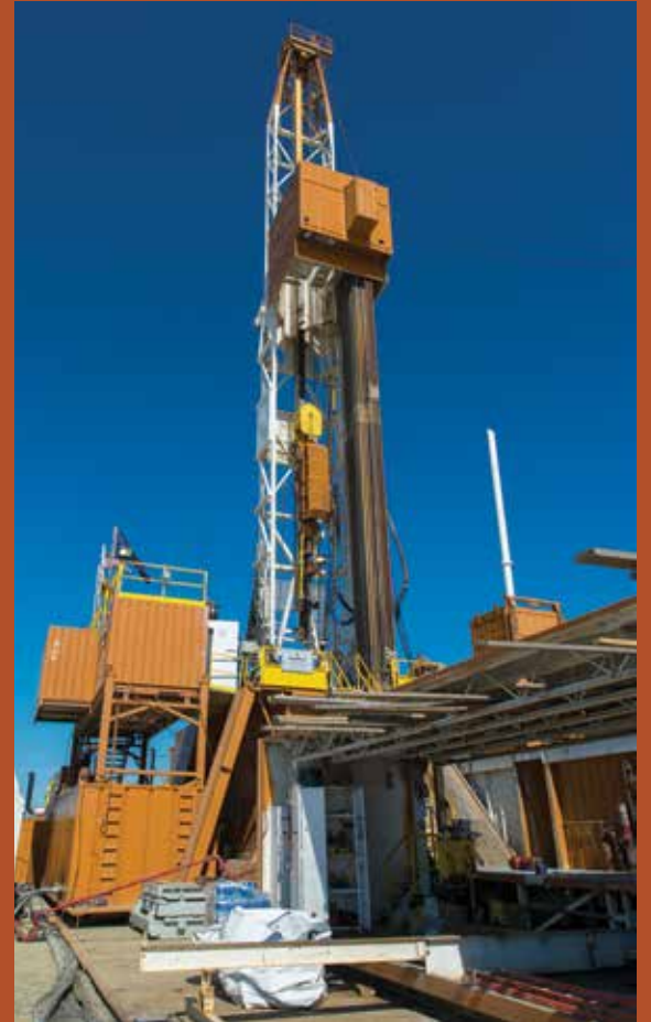
The Toghothelle drill site, a 2016 partnership between Doyon and CIRI. Photo by J. Irwin.
