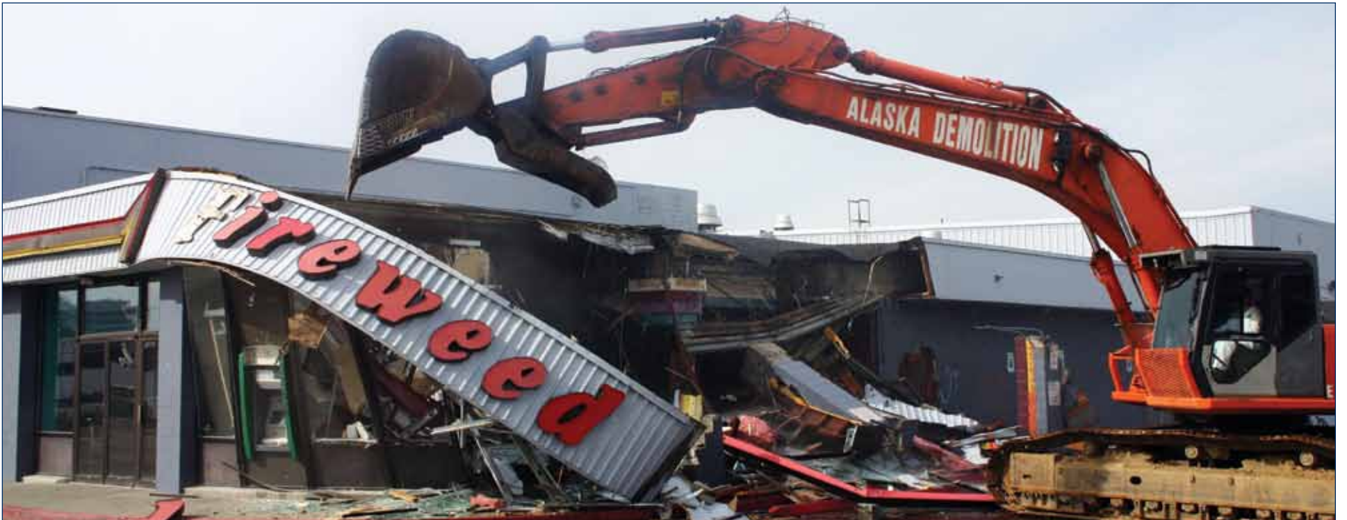
Anchorage contractor Alaska Demolition tears down the Fireweed Theater building in midtown Anchorage on Aug. 26. The site is anticipated to be transferred to CIRI Land Development Company in late October.
