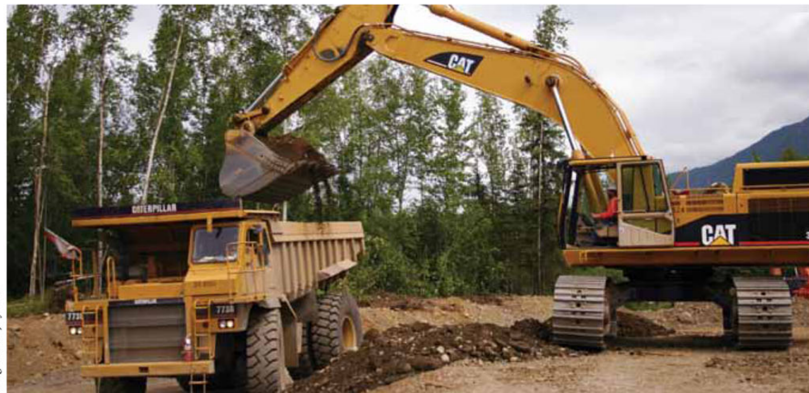
The sand and gravel extraction project on Eklutna land in Birchwood, Alaska, won a Tileston Award on July 21. The project is a partnership between CIRI and Eklutna Inc. and is operated by Wilder Construction.
