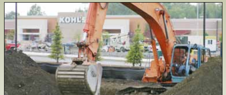
A new Olive Garden is being built at Tikahtnu Commons. CIRI Land Development Co. is teamed with retail developer Browman Development Co. to develop Tikahtnu Commons on 95 acres of CIRI land in northeast Anchorage.
