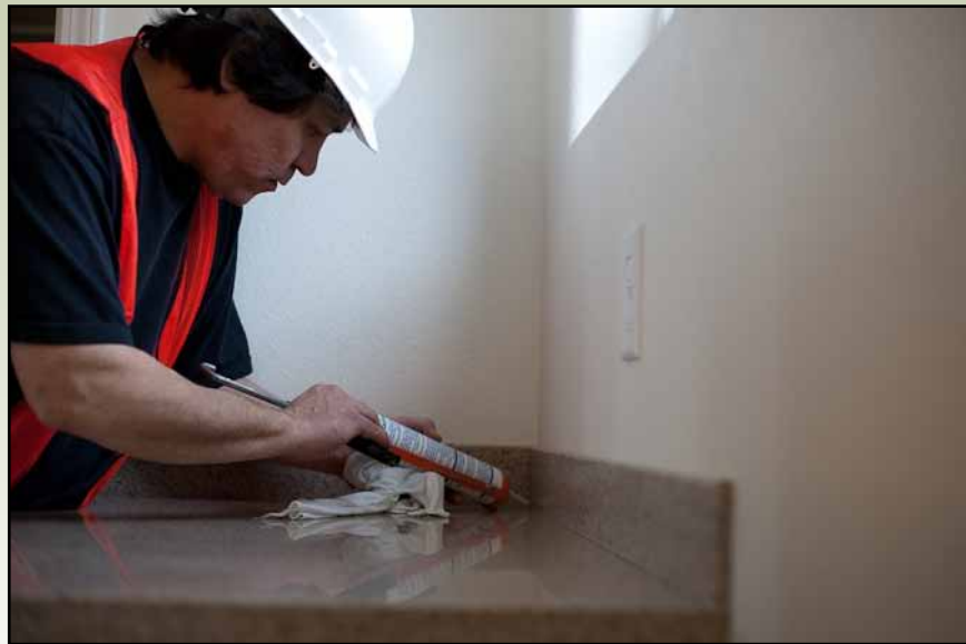
Finishing touches are applied to a Loussac Place home. Applications are now available online at www.cookinlethousing.org for rental homes at Loussac Place, located between A Street and C Street off of 20th Avenue.
