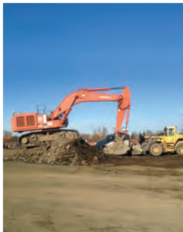
➤ Crews with Davis Constructors & Engineers, Inc. begin site preparation work for the Fireweed Business Center. Photo by Jason Moore.
