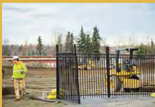
Construction crews prepare Fireweed Business Center site for winter shutdown. Photo by Joel Irwin.
