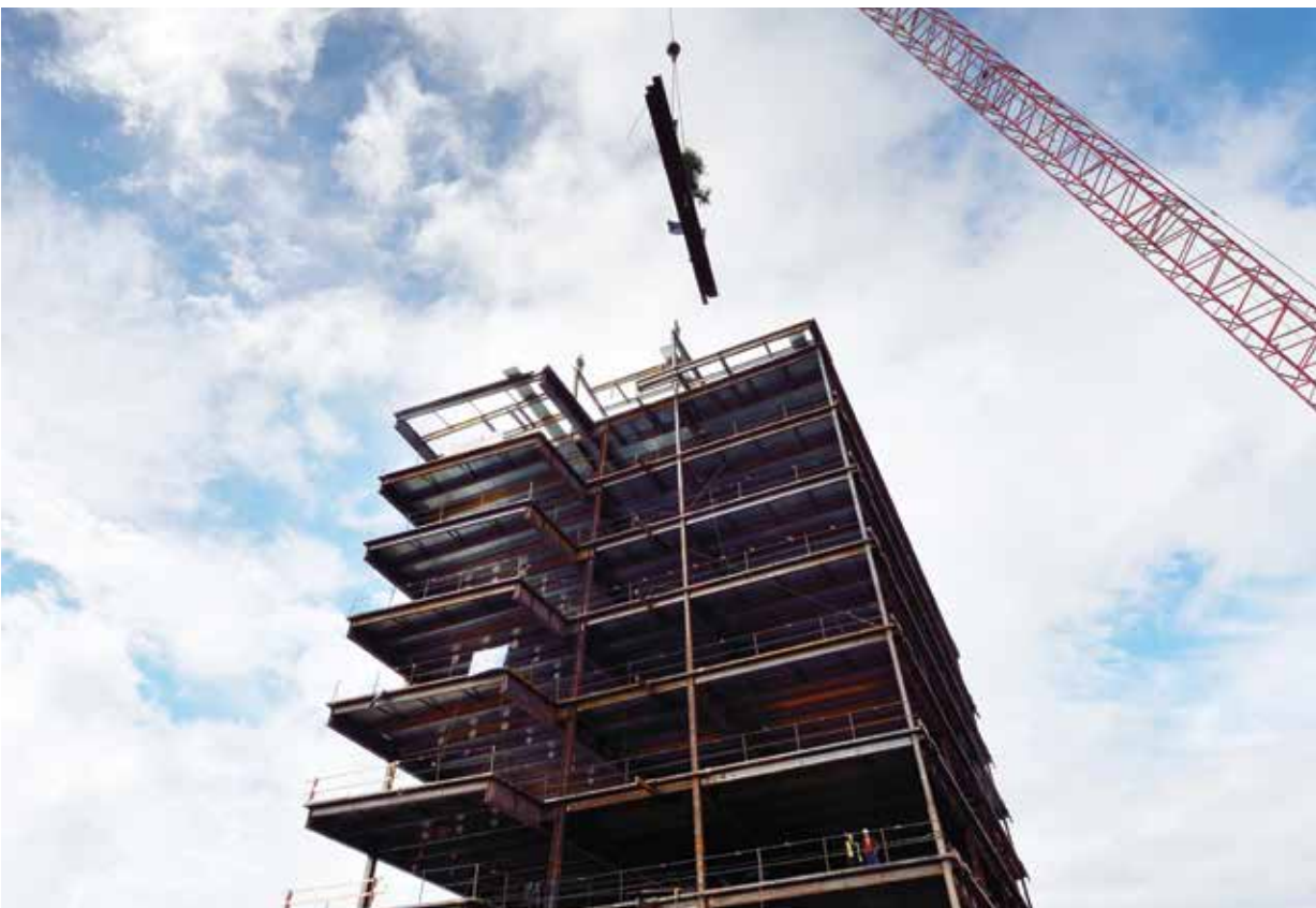
➤ The last steel beam being hoisted to the skeleton frame of the Fireweed Business Center. Photo by Jason Moore. See more photos on page 4.
