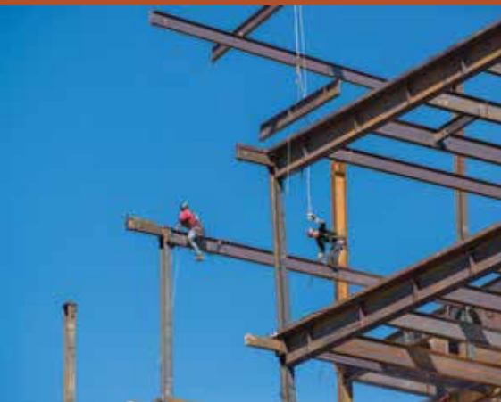
Construction of the Fireweed Business Center. Photos by Jason Moore and Joel Irwin.
