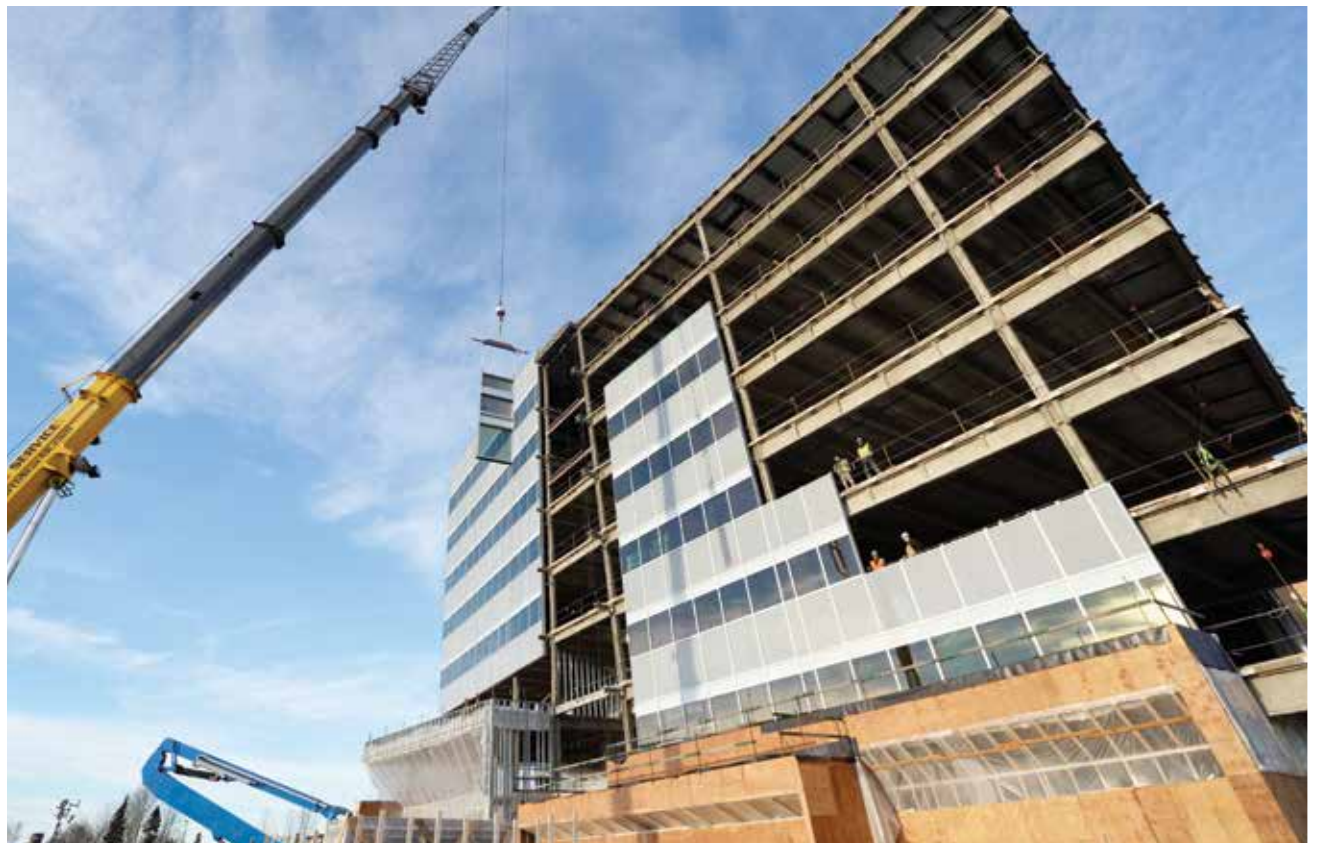
A glass panel is lifted into place on the Fireweed Business Center. Photo by Joel Irwin.
