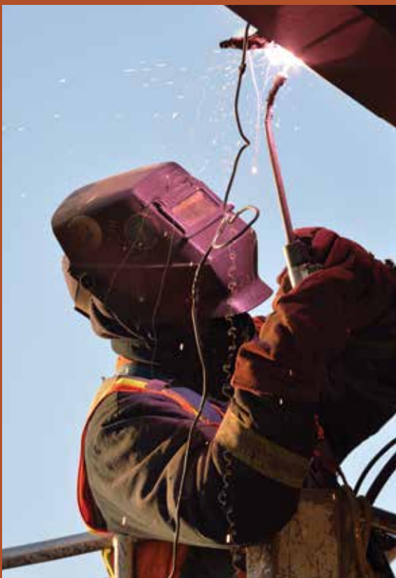
Sparks fly as the finishing welds are completed on the structural supports. Photo by Jason Moore.
