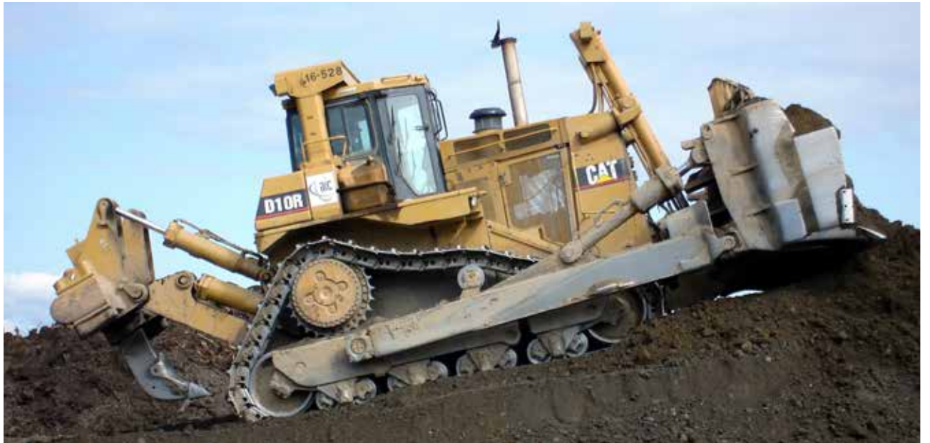
☛ An Alaska Interstate Construction bulldozer working on construction of Anchorage's Tikahtnu Commons in 2007.
