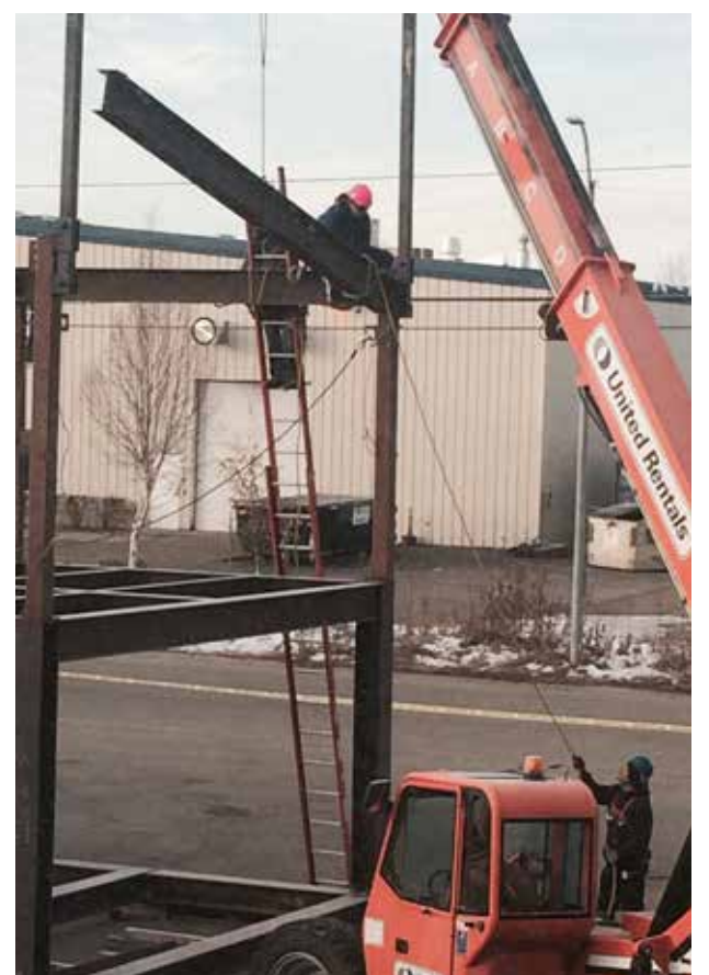
» Students in CITC's new ironworkers pre-apprenticeship training program practice their new skills. Courtesy of Cook Inlet Tribal Council.
