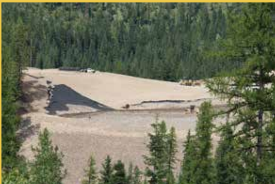
➤ The waste will be placed and compacted to prevent air, water and soil contamination. Photo by Jason Moore.
