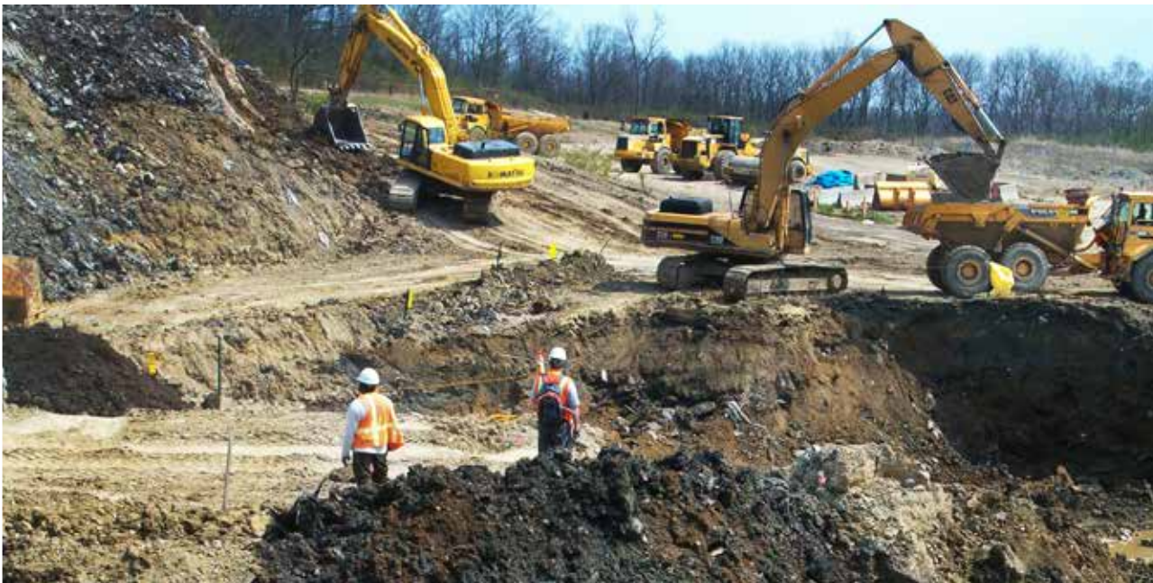
Portage is an expert at environmental cleanup work, which includes excavating, loading and hauling waste, and accepting, placing and compacting that waste at separate disposal sites. Photos courtesy of North Wind Group.
