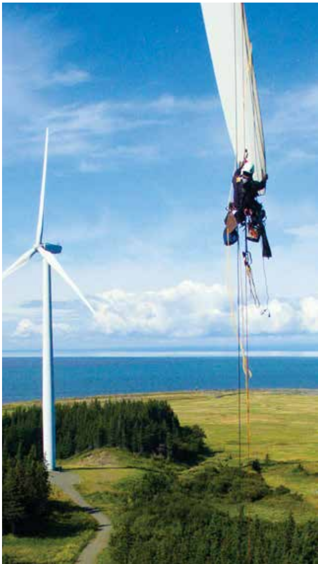
➤ A worker performs turbine blade repairs at Fire Island Wind. Photo by Jason Moore.
