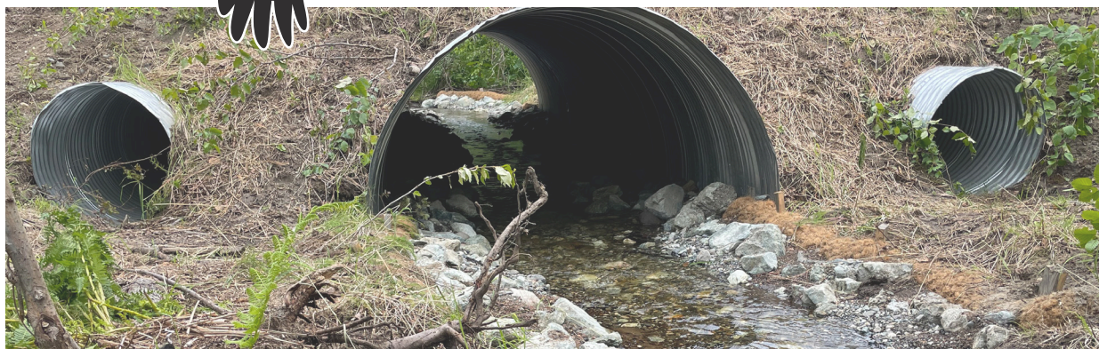
Culvert-replacement projects, such as this one in Tyonek, are aimed at increasing and improving salmon habitat. Photo courtesy of TTCD.
