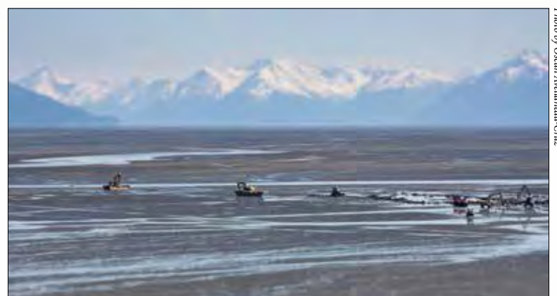
Wasilla-based Cruz Construction workers help install a submarine transmission cable linking Fire Island to Anchorage in June.
