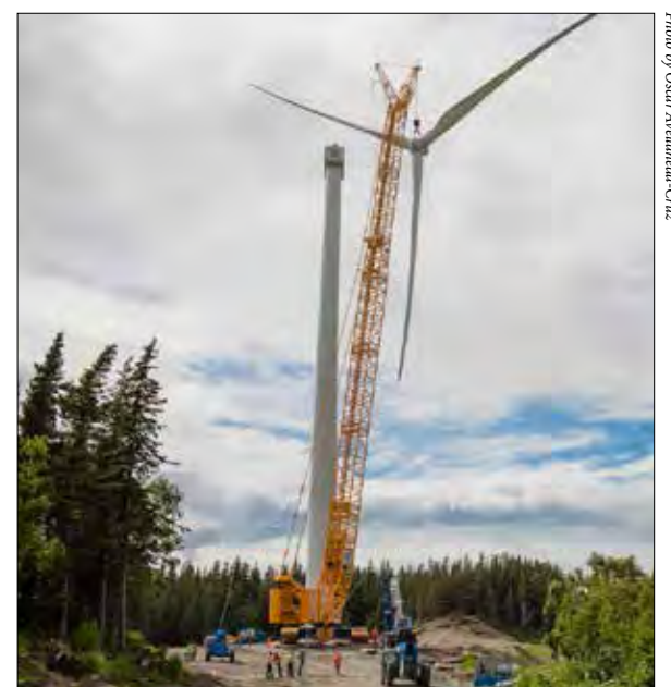
Workers use a crane to lift a rotator assembly into position atop a turbine tower on July 10.
