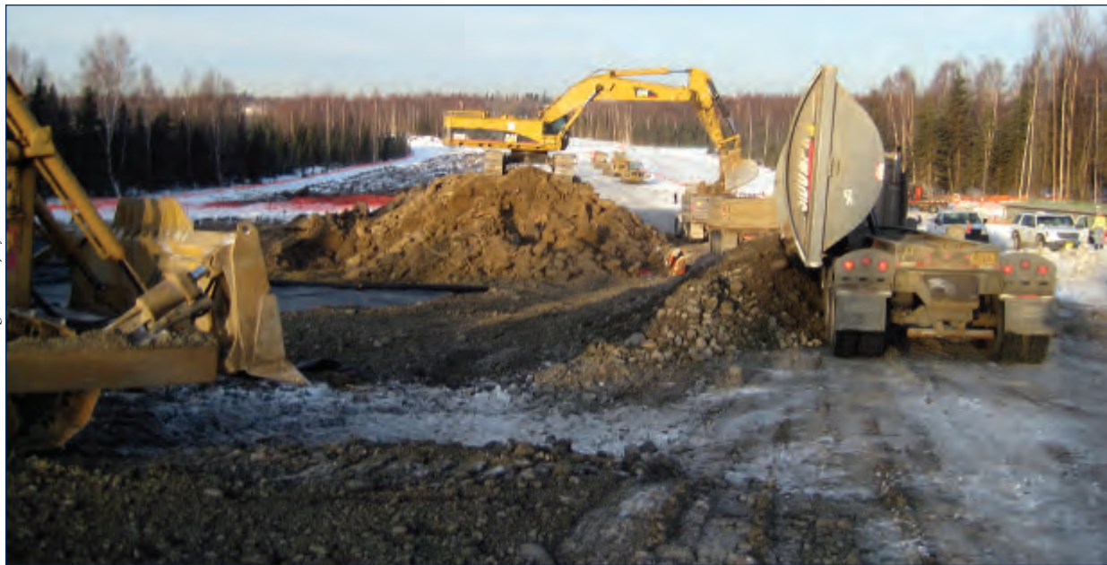
Alaska Interstate Construction LLC crews construct Martin Luther King Ave., a new Anchorage road linking Boniface Parkway and Elmore Rd.
