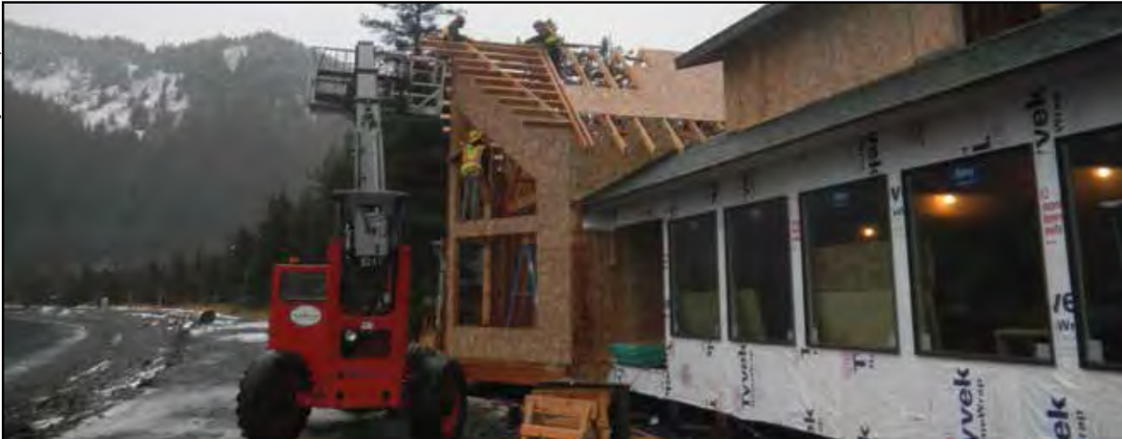
Crews work on constructing the roof of the new Kenai Fjords Wilderness Lodge overnight building.
